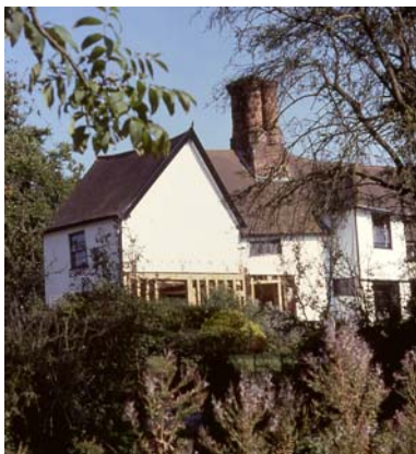
Clock House, Stonham Parva - timber frame repairs and extension to a Grade II Listed farmhouse
