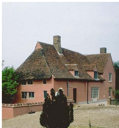
Abbas Hall, Great Cornard - timber frames repair and refurbishment of 13c. aisled hall, Grade I Listed
